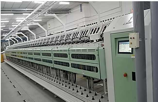
A view of new “LMW-LF 4280A”-Simplex Machine installed in our Unit-II at Subramaniyapuram.
