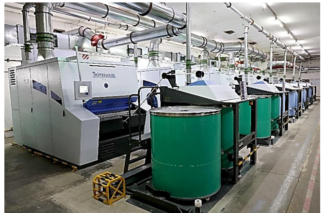
A view of new “Trutzschler – TC 15” Carding Machine installed in our Unit – I at Rajapalayam.
