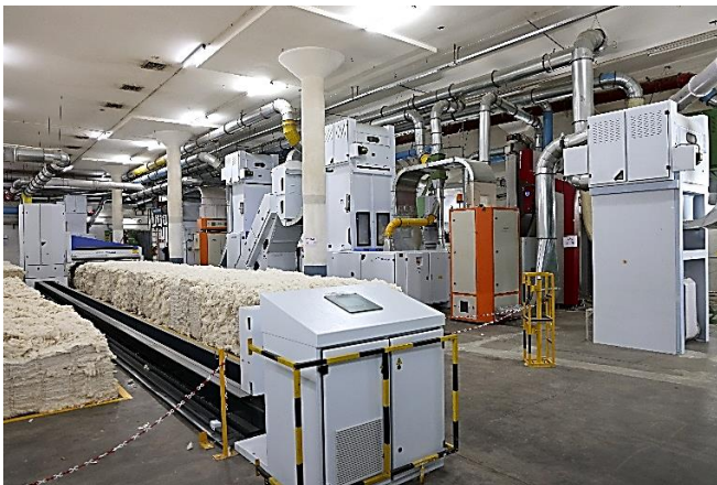
A view of new “Blendomat Trutzschler” Automatic Bale Opener Machine installed in our Unit – I at Rajapalayam.
